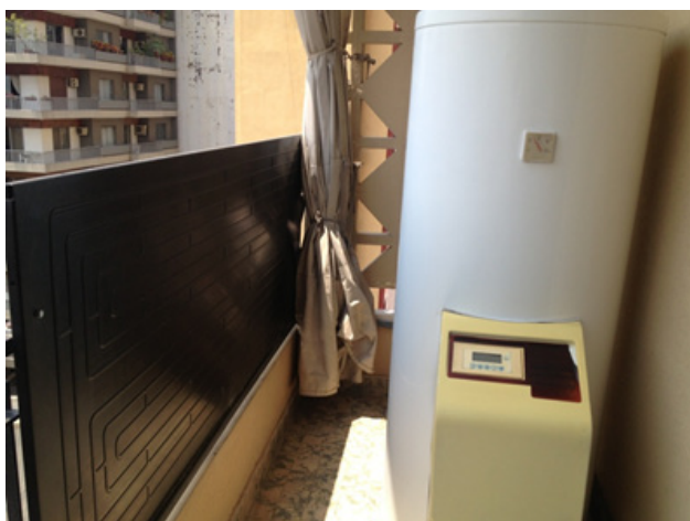
Figure 14: solar thermodynamics installation
