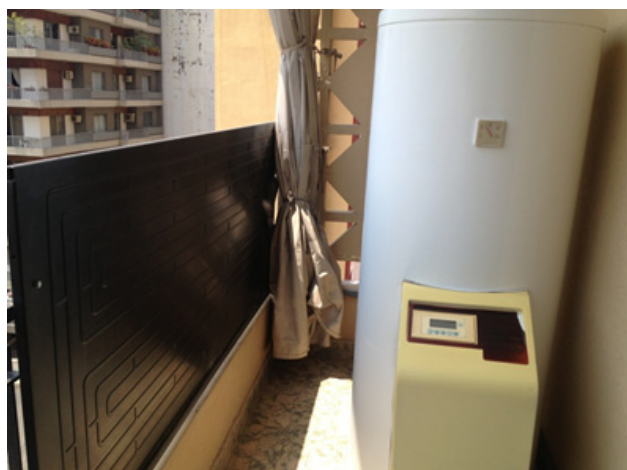
Figure 14: solar thermodynamics installation
